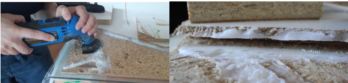
Figure 13: Front corner piece levelling and creation of a groove to insert the plywood consolidation piece.
